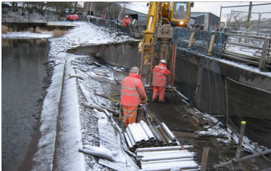
Figure 4. Installation of TaM holes over central spillway showing reservoir water level maintained during the works
