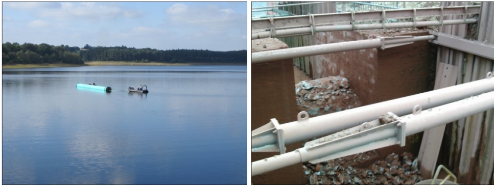
Figure 5: View of the intake section of siphon pipework being floated across Eccup ESR (left) and cutting through the brick pillar for the siphon pipe (right).
