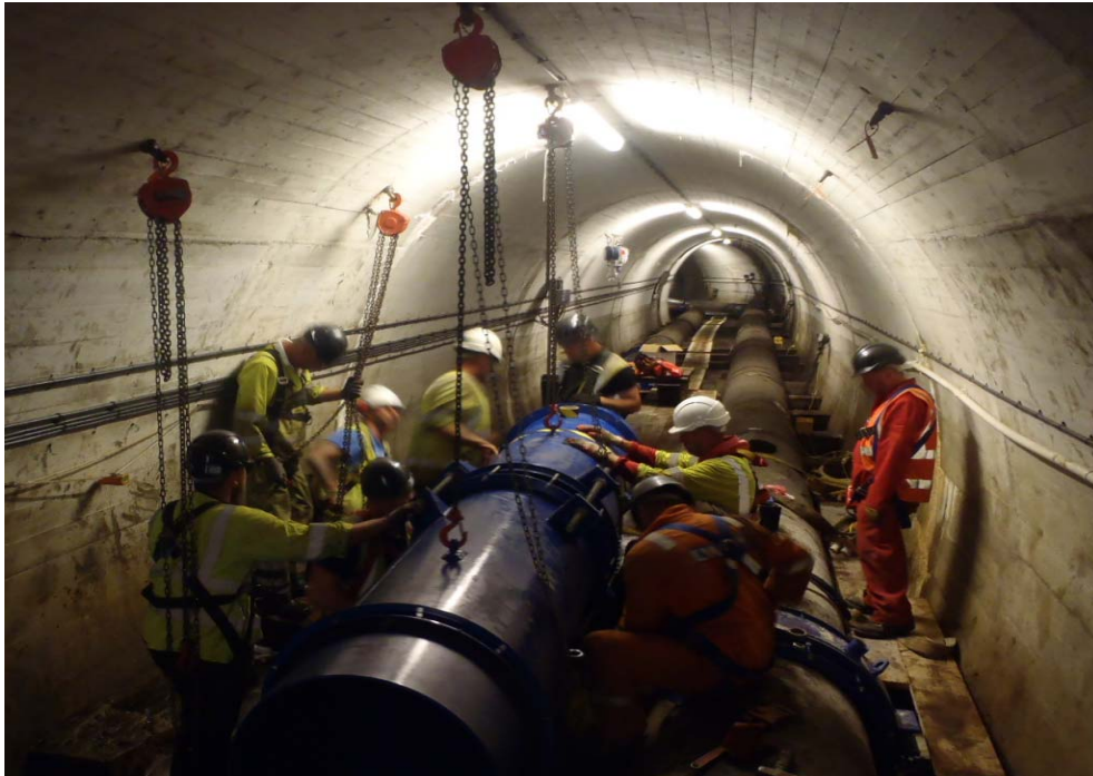
Figure 5. Lifting in the new section of pipe to replace the failed section
