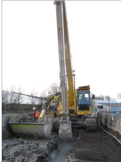
Figure 3. Installation of slurry trench cut-off wall with vacuum excavator removing arisings from skip
