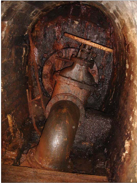
Figure 10. Existing Drawoff Valve in Downstream Tunnel
