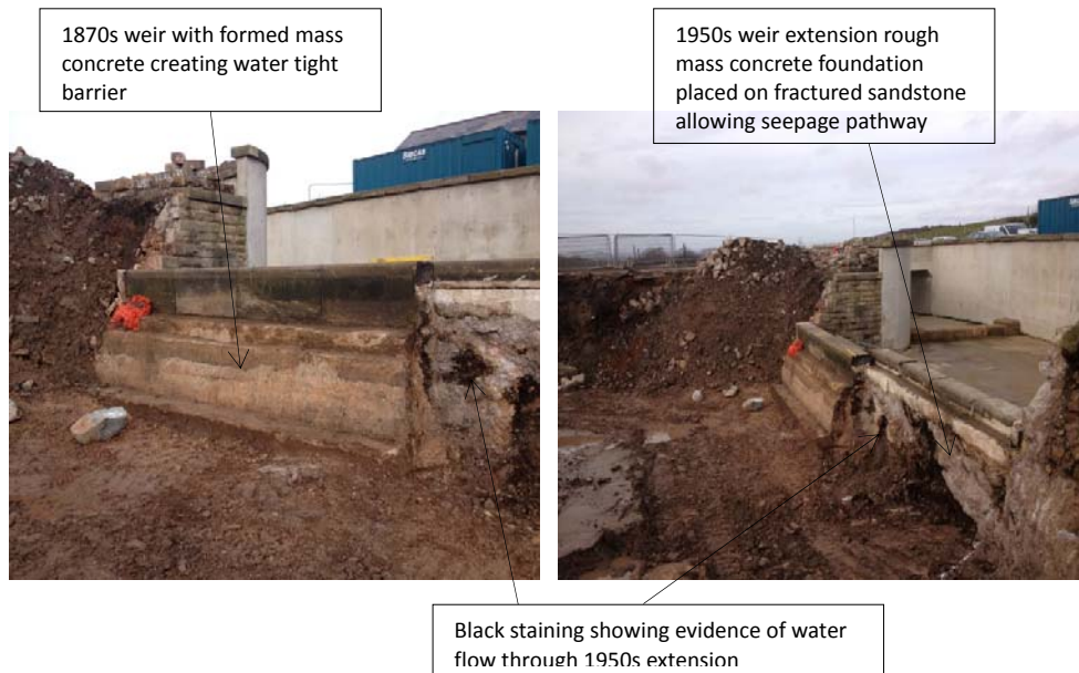
Figure 4: 1870s weir and 1950s weir extension showing evidence of seepage
