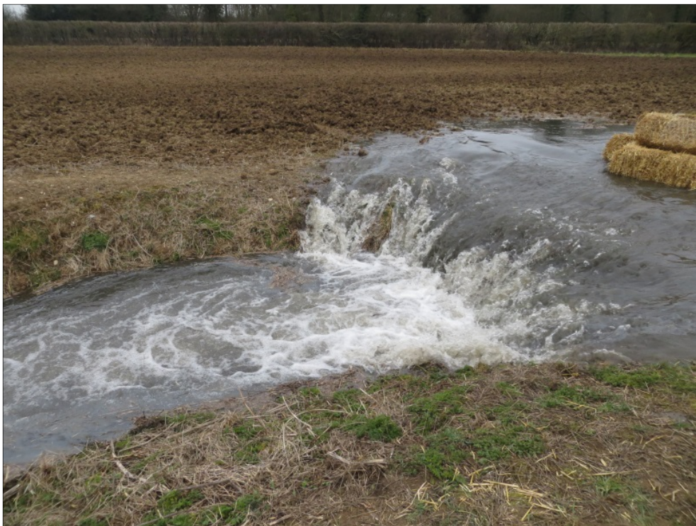
Figure 6. Overtopping of field access culvert
