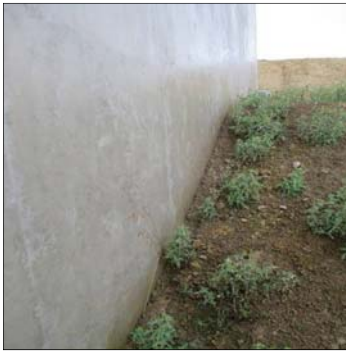
Figure 6. A newly constructed reservoir, backfilled contrary to specification, without drainage membrane. The omission of a membrane allows the backfill to support an elevated ground water level with potential to introduce contamination if a movement joint fails or a wall cracks.
