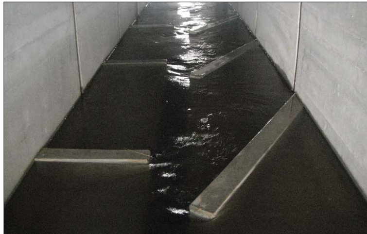
Figure 8. Baffles in Crayfish Culvert (Culvert #1)
