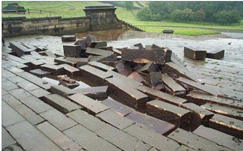
Figure 2 - Damage caused to spillway invert in 2002
