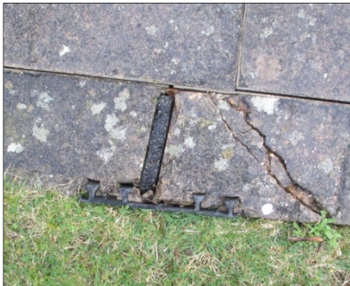
Figure 7. A further illustration of poor workmanship where the expansion joint, unusually employing rear guard water stop, has moved during construction. Furthermore the exposed detail allows ingress down the wall joint and into the reservoir.
