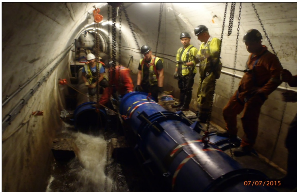
Figure 4. Flow discharging at the removed section of the scour main
