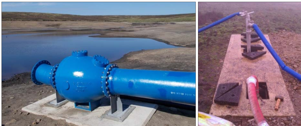
Figure 2: View of intake NRV (left), and the siphon crest priming arrangement (right).
