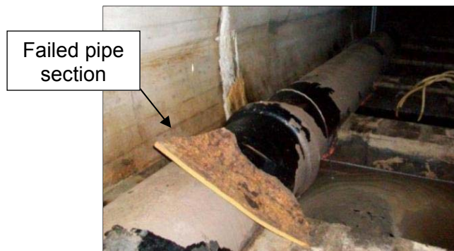
Figure 3. Section of the pipe that burst from the underside of the pipe
