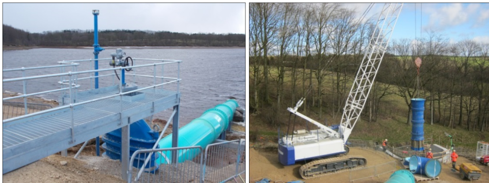
Figure 4: View of Eccup ESR siphon gate valve (left) and terminal submerged discharge valve (right) during construction.
