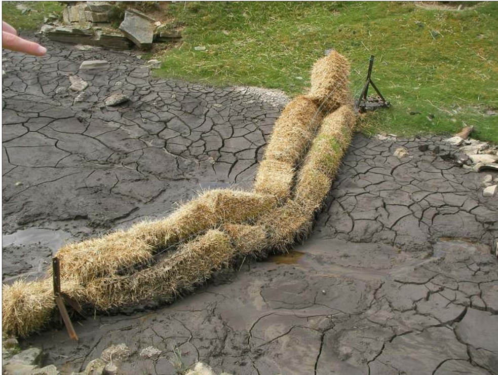
Figure 3. Inadequate means of treatment in place
