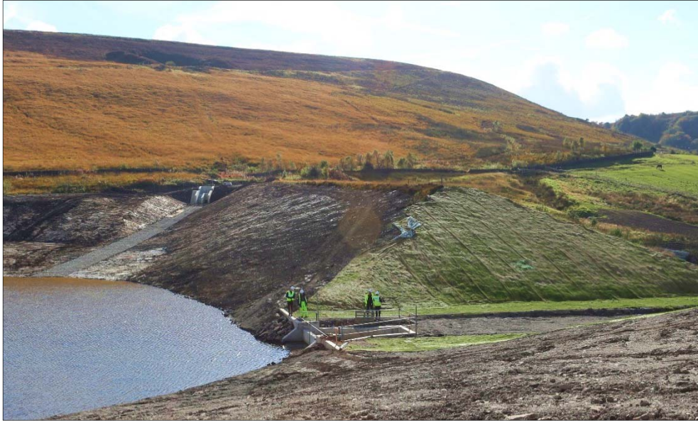
Figure 2. Completed notch cut through Sunnyhurst Hey embankment (centre right) with new concrete inlet screen structure (background, centre left) and new concrete outlet weir (centre bottom).
